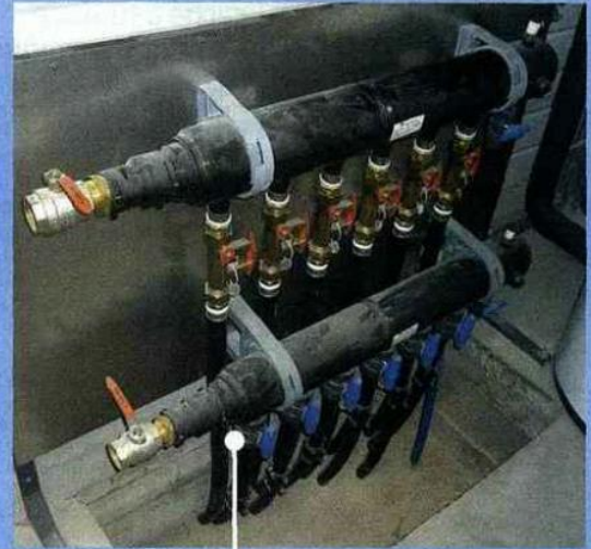
Six boreholes 100 meters of depth The boreholes contain double-U pipes of 40mm diameter. The water (without Glycol) flowing in closed circuit in these pipes is the same as that flowing through the fan coil units in geocooling mode.
